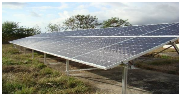
Figure 3: Photovoltaic Generator 7.5 kWp.
