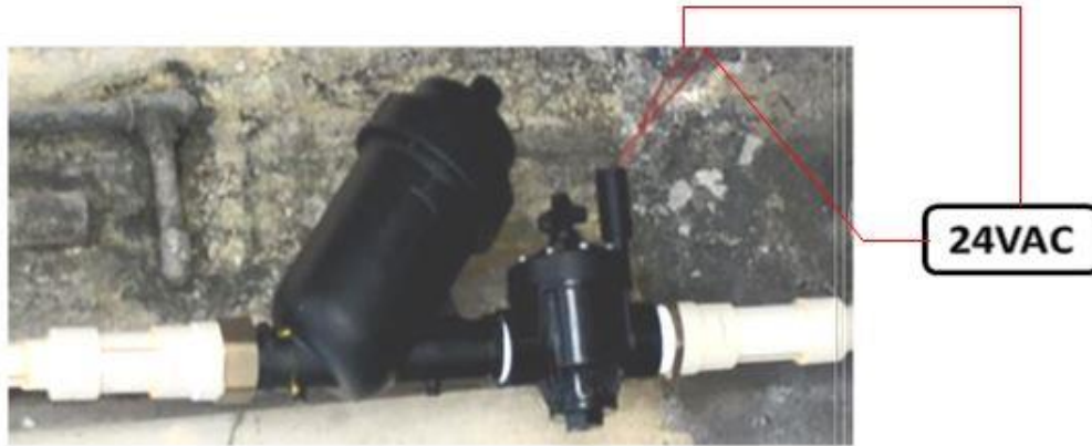
Figure 2. Solenoid Valve connected with power supply installed at site
