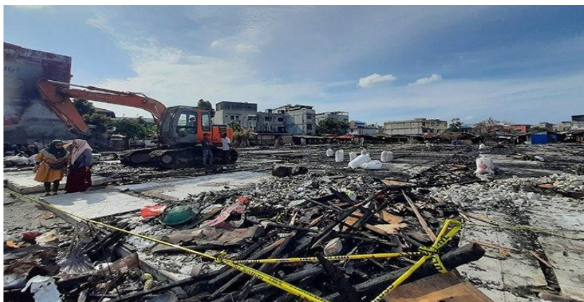
Figure 7. Debris from the Fire
